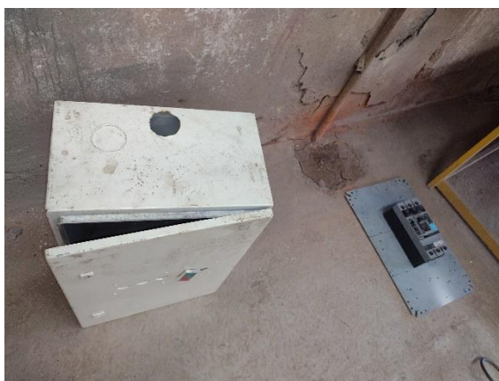
Figura 15. Tablero e interruptor a instalar
